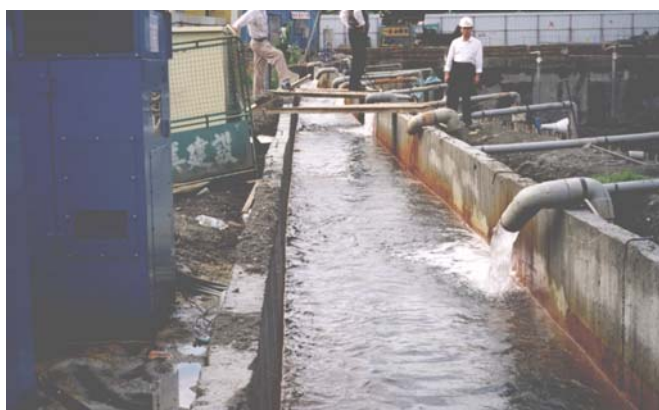
Fig. 7 Deep wells in operation
