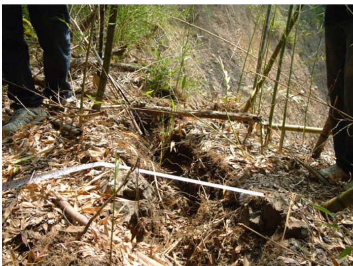
(a) Tension cracks at the upper slope of Makino bamboo forest slopland
