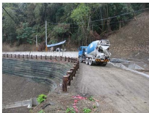
Fig. 7 The completed embankment at the experimental site and subjected to traffic loading
