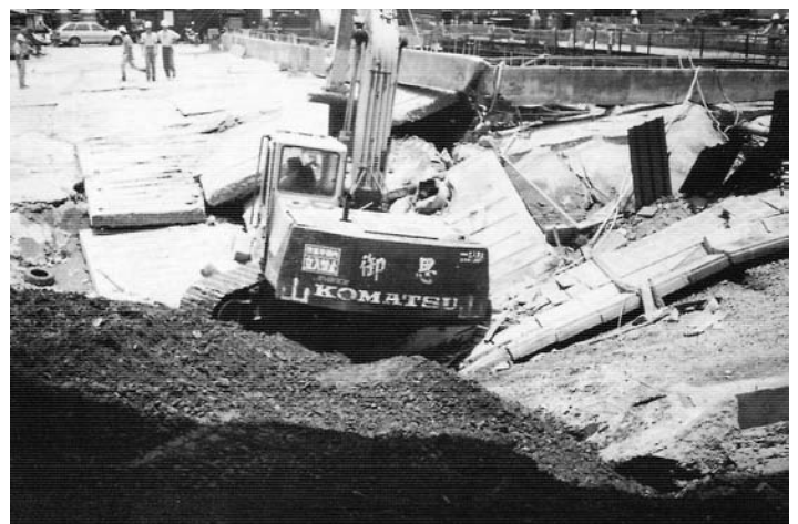
Fig. 7 Emergency fill for ground settlement near shaft A
