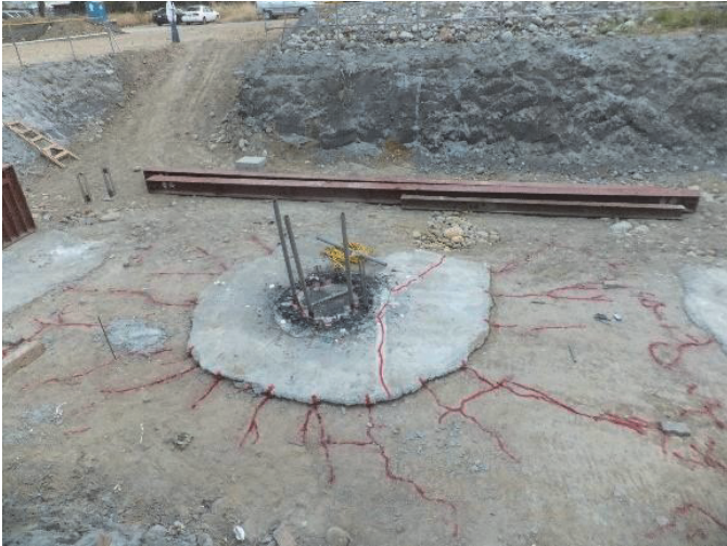
Fig. 18 Ground surface cracks around the test pile
