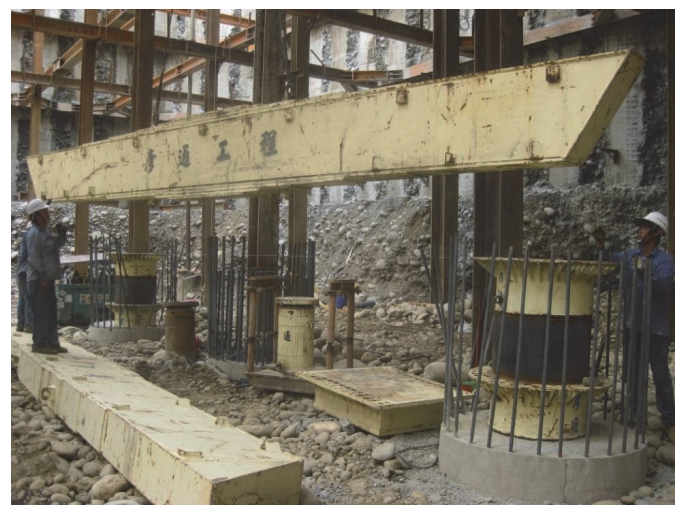
Fig. 14 An uplift pile loading test conducted at the bottom of basement excavation
