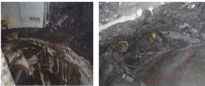
Fig. 9 Swelling pressure encountered at the top and bottom of the tunnel cross section ( K = 0.5 )
