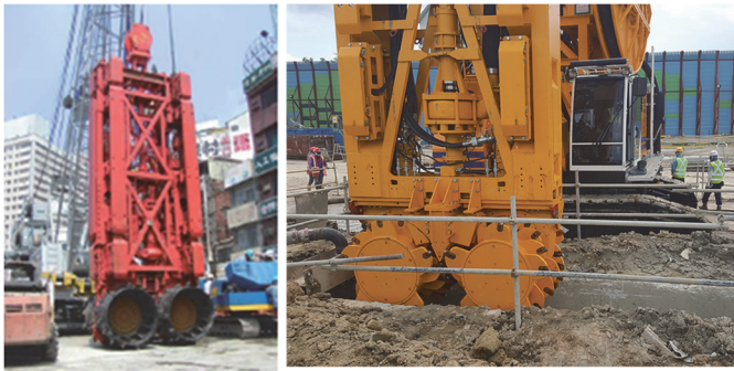
Fig. 4 EXM and similar trench-cutter machines used for diaphragm wall construction of O5/R10 station
